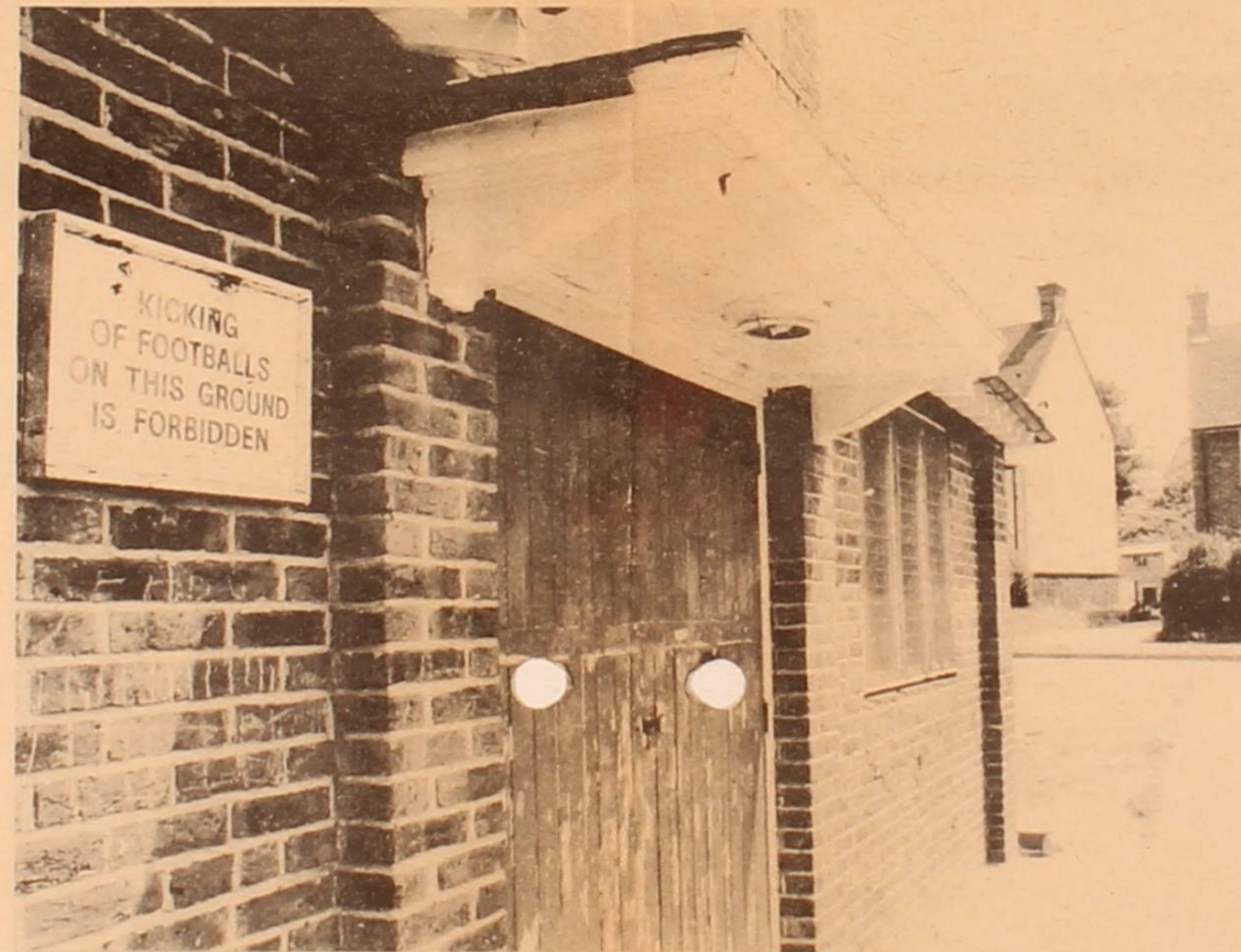
ITS WINDOWS GRILLED TO BEAT VANDALS, ITS PAINTWORK PEELING, THE COMMUNITY CENTRE IN MOULSECOOMB PRESENTS AN EXTERIOR AS BLEAK AS ITS INSIDE IS GRIM. NOT SURPRISINGLY, THE HALL IS LITTLE USED. YET, INSTEAD OF JUST HOUSING BINGO SESSIONS, IT COULD SERVE AS FOCUS FOR THIS PART OF THE ESTATE.
