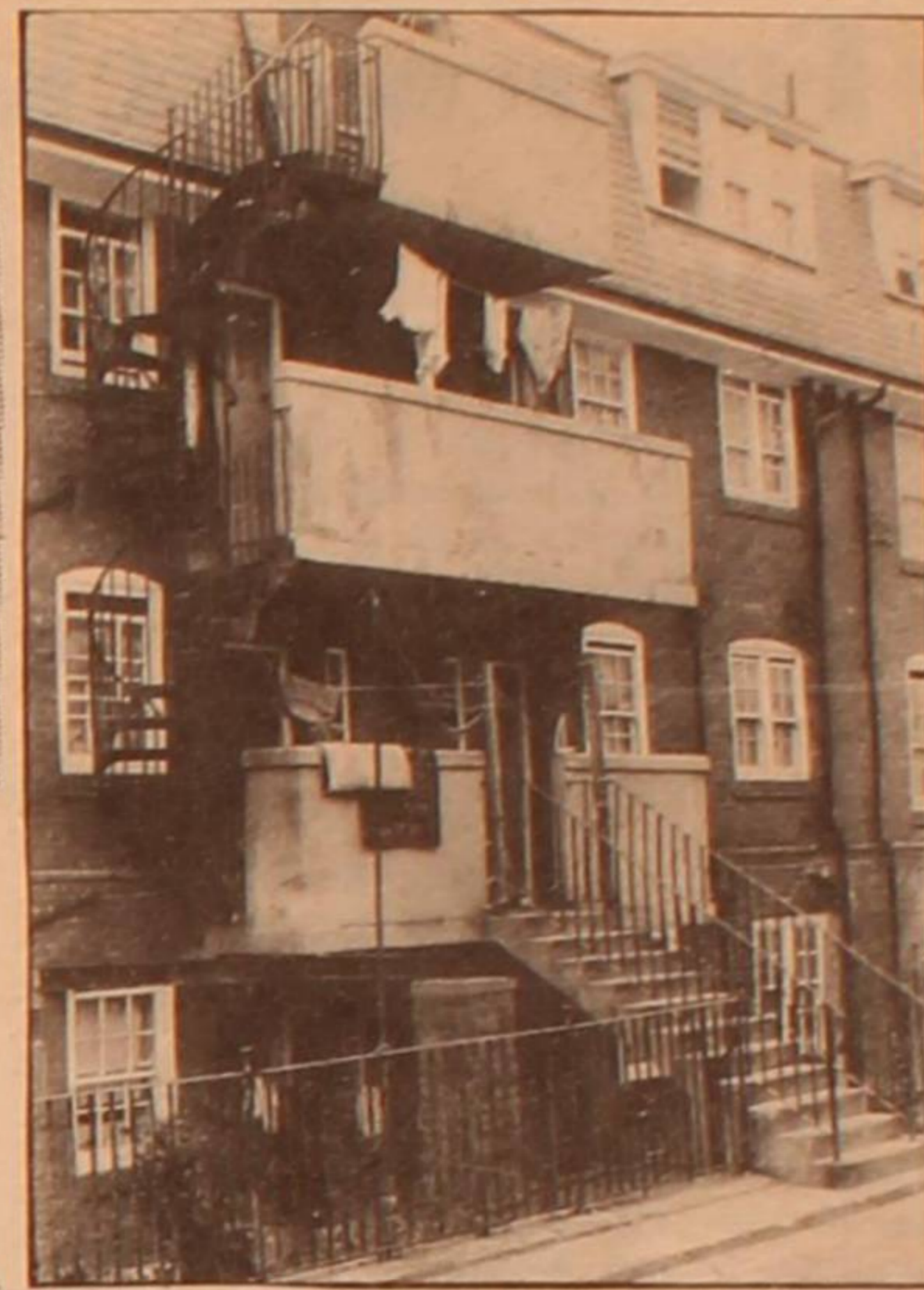
Milner Flats-gutters filled with growth, mould on bedroom walls. Three families of 'boat people' housed here. There's only one word you can say about it - a resident told Brighton Voice.
